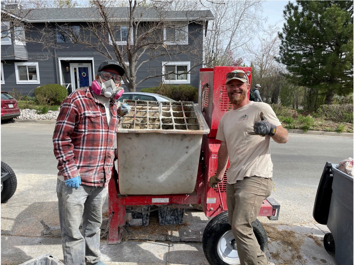
Phelan Dalton (L) and Eamonn McNaughton (R) provided volunteer supervision for the construction the hempcrete wall in Boulder. Photo by Jean Lotus
